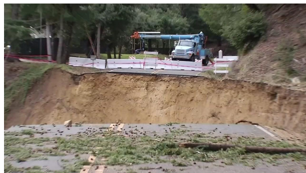
Annual storms often result in damage to and closure of local roads within the County. The 2016/2017 storm season was especially damaging mountain roads, resulting in the temporary closure of many roads, such as Highway 35 (pictured above).
