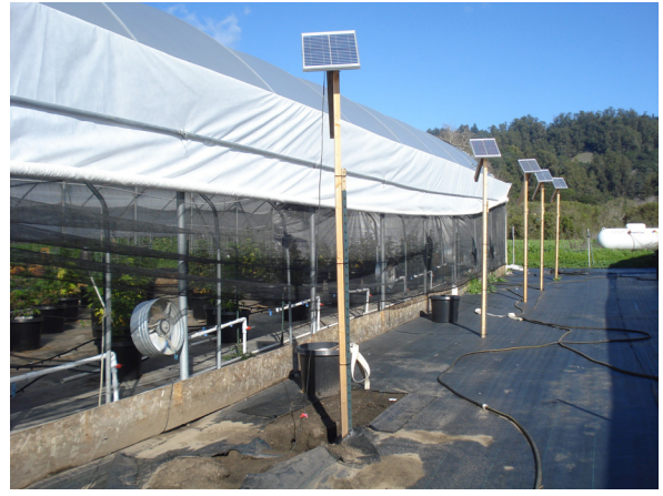
Some existing grows within the County support environmentally friendly cultivation methods; one approach is to provide electricity needs for fans and other motors through solar panels and batteries.
