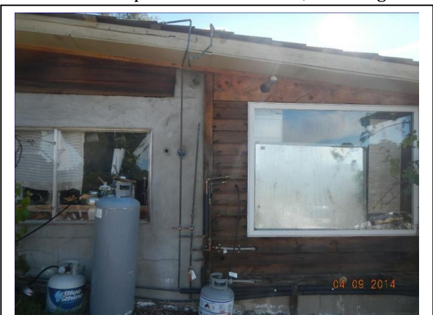
A common hazardous practice conducted by some existing unlicensed cannabis sites is the unsafe storage of toxic, flammable, and explosive materials and equipment.
