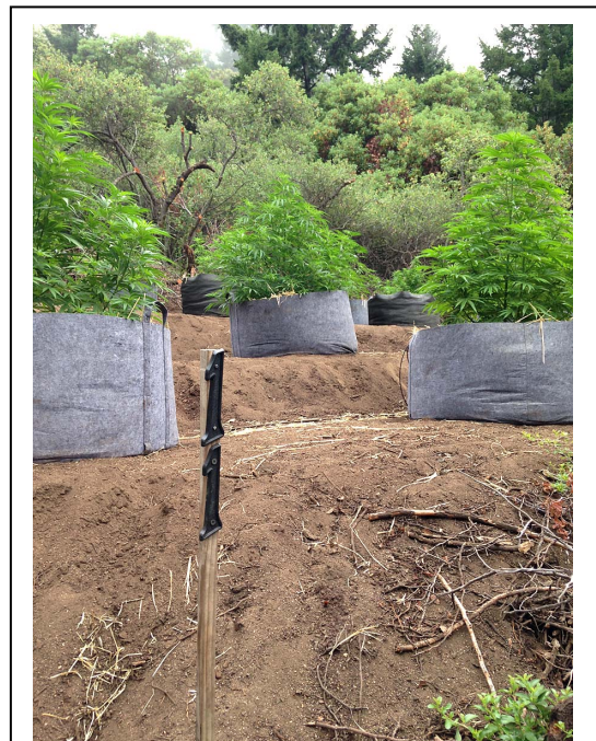
Site preparation activities for outdoor grows, such as vegetation clearing and grading, cut and fill, and building support facilities (e.g., roads, water supply facilities), could increase the potential for erosion or landslides.
