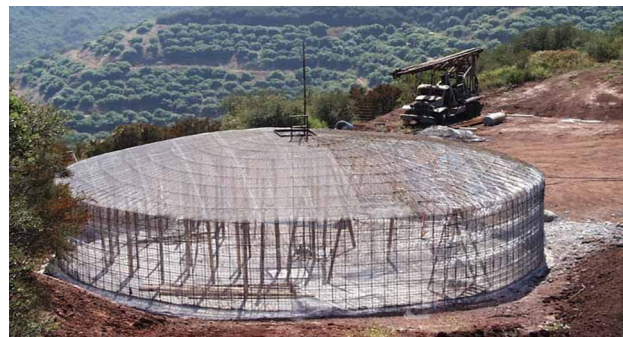
For F-1 Factory Industrial classifications, the Fire Marshal has determined that up to a 120,000-gallon storage tank or more may be required for adequate water storage. Such a tank is roughly 30 feet in diameter by 25 feet tall. Multiple smaller tanks can also be co-located on the site to meet the storage requirement. Cannabis drying sheds and greenhouses would be considered F-1 occupancies. Sprinklers may be required, including for cannabis drying sheds and greenhouses, depending on whether located in a rural area not served by municipal water, and whether employees work within buildings.
